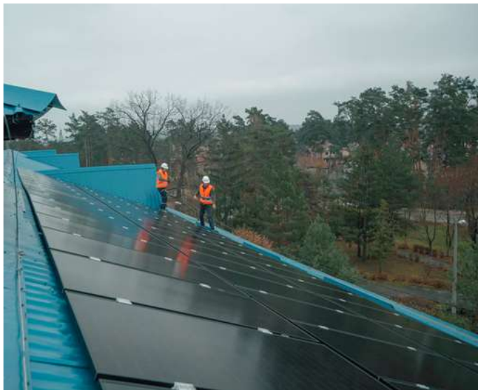
Solar power plant in Irpin city. Source: Energy Act for Ukraine
