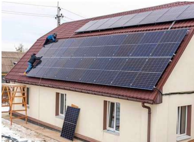
Solar panels on the roof of Horenka hospital. Source: Greenpeace
